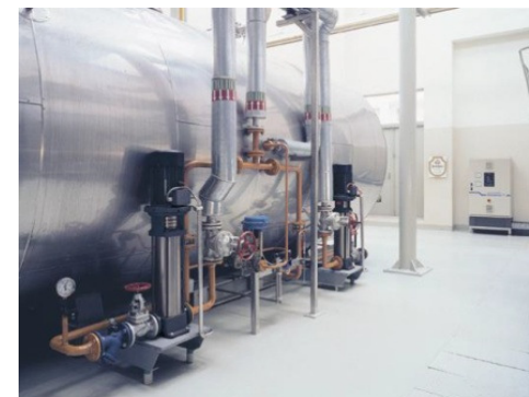
Boiler feed water
