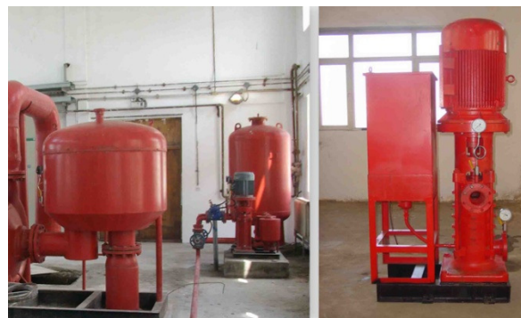
Fire fighting system
