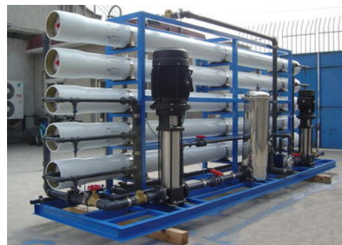
Water treatment - RO system
